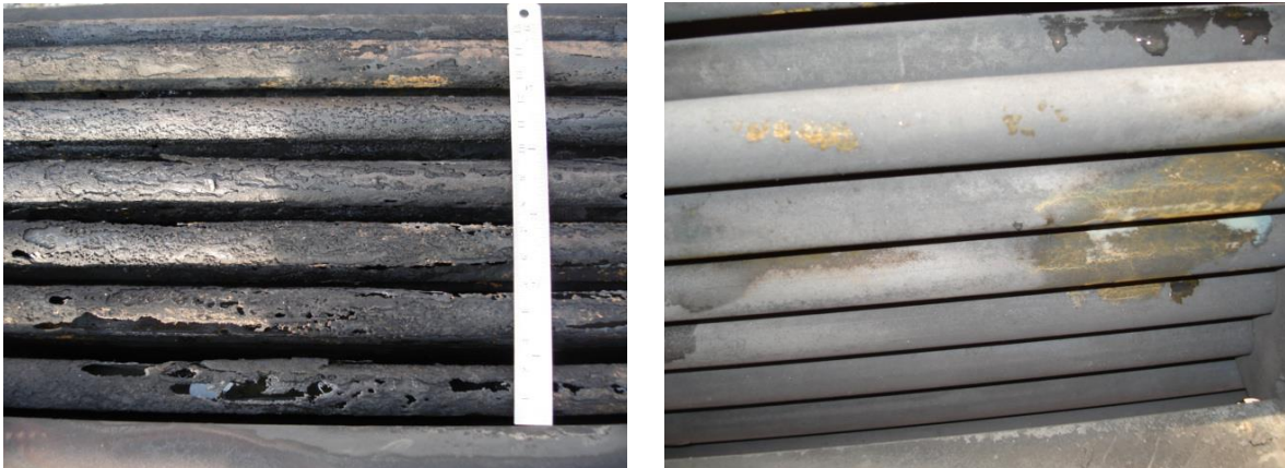
Figure 6 Sour water stripper reboiler (carbon steel) top row tubes (left) and bottom row tubes (right)
